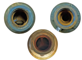
Inlet and outlet of worn pressure regulators.
